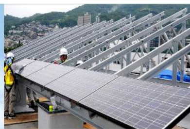
SOLAR POWER PLANT & STRUCTURE
